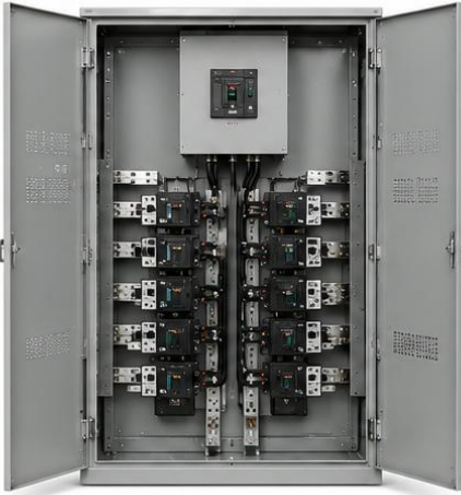
MDP PANEL (MAIN DISTRIBUTION PANEL)
